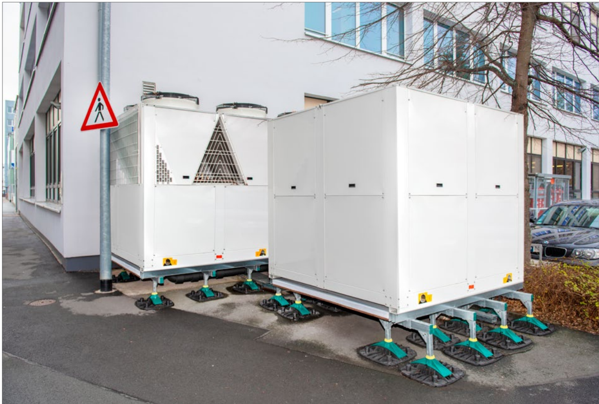
Our new industrial cooling system
